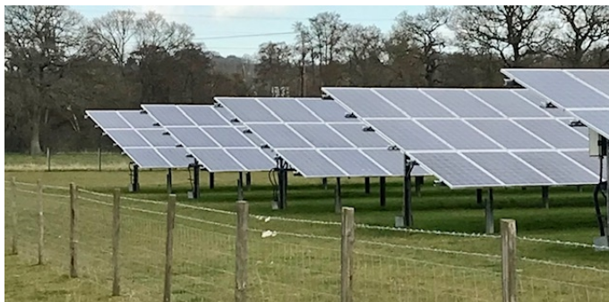
Figure 6: PV panels at Partridge Farm solar farm, Aldington, Kent.
